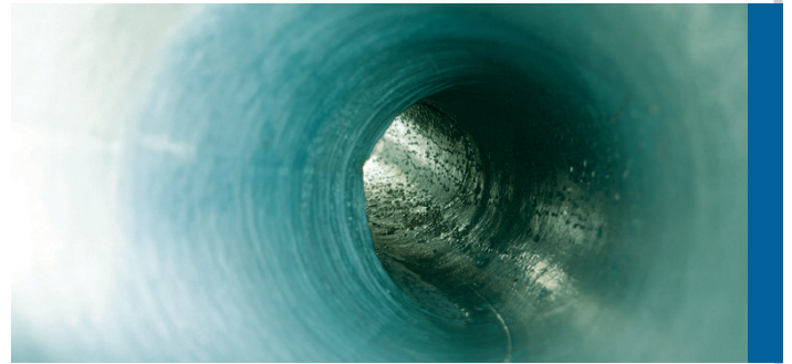
AFTER: CIPP lining systems combine liner materials with resins designed and formulated to address the demands of your piping system.
