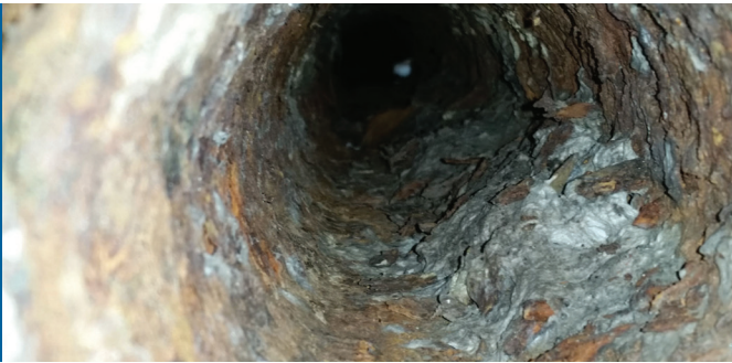
BEFORE: In many cases, water and sewer pipes that appear to be beyond repair can be CIPP lined and fully rehabilitated.
