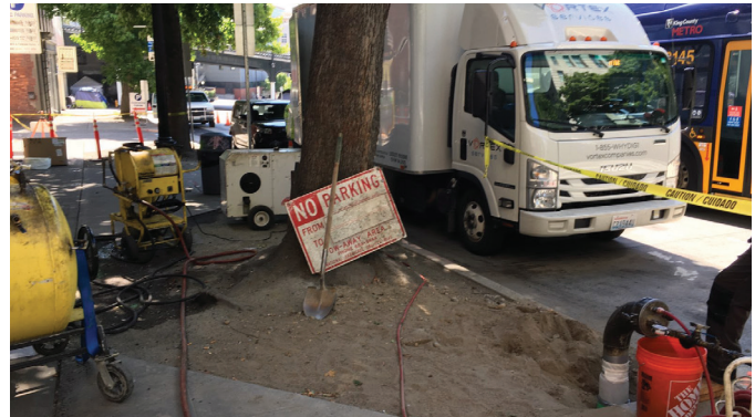
With limited access due to the trees and sidewalk, the lateral and main could only be replaced by the Quad-Cure® CIPP method.
