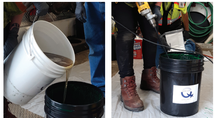
Quad-Cure® 3100 resin system being mixed prior to wet out of the liner.
