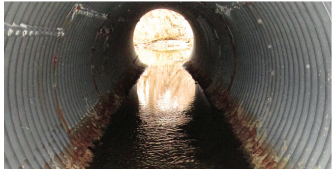
78" CMP was corroded and failing.
