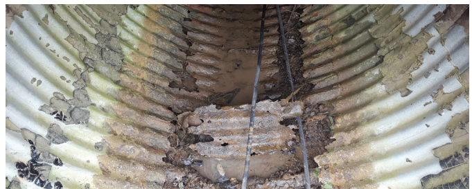
This old CMP culvert was completely corroded through in many areas.
