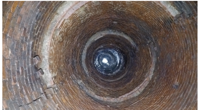
Multiple baffles had to be removed prior to rehabilitating the noticeably cracked 125' deep manhole.
