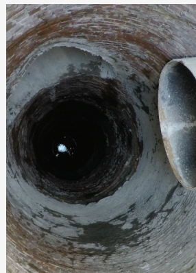
Before: Total restoration was required to bring the sewer back to original operating conditions.
