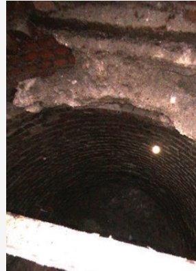
15 concrete baffles, like this damaged one shown, had to be removed from the manhole.
