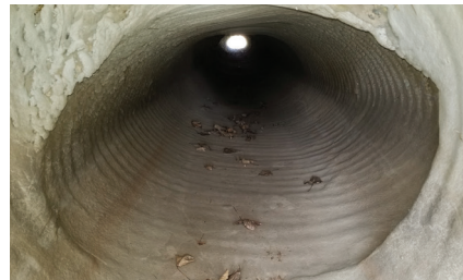
October 2017 No signs of joint failure or ovality as depicted in the host pipe. Structural GeoKrete liner is intact and continues to provide corrosion protection.
