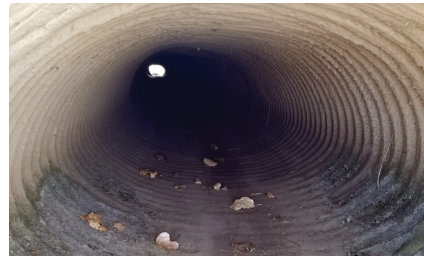
October 2017 Section of pipe where partial collapse existed remains in excellent shape after it was structurally relined with GeoKrete.
