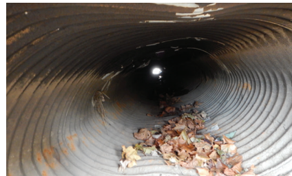
July 2015 Pipe sections showed signs of partial collapse.
