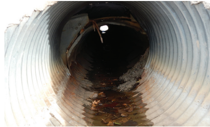
July 2015 Complete joint failure with pipe suffering from severe ovality, I&I and threat of total collapse.
